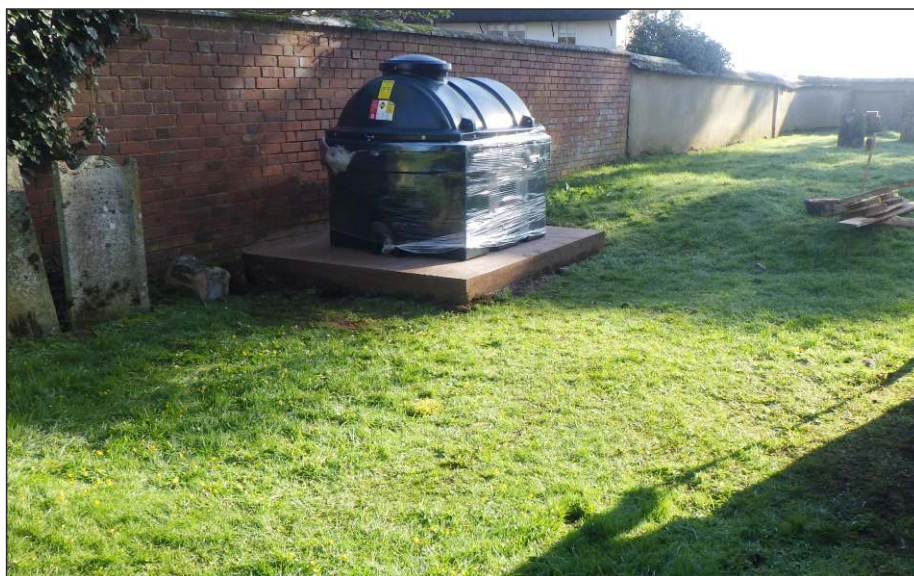
Plate 1: General view looking northeast at area of new oil pipe trench prior to excavation
