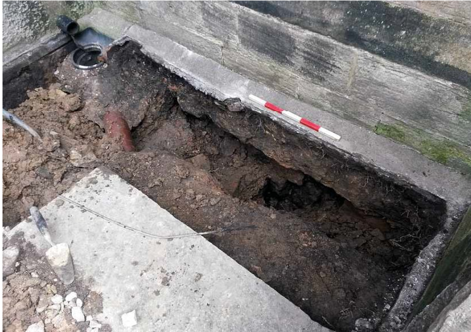
Plate 5. Test Pit 3, showing poor condition of foundations, looking north-east
