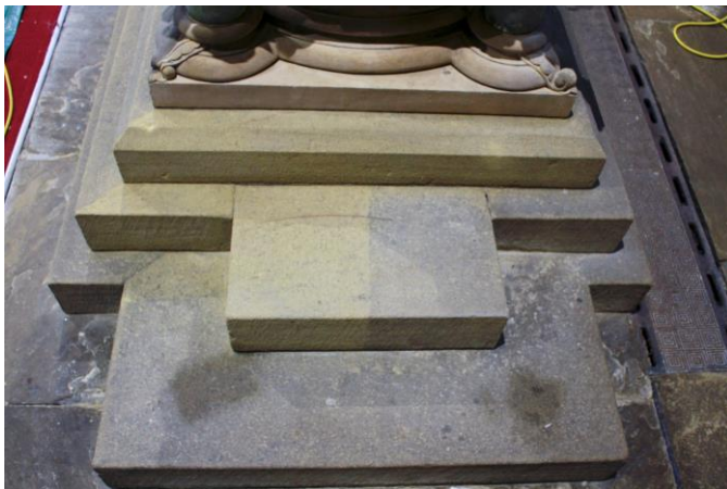
A cleaning contrast to the middle step, showing the subtle level of difference in cleaning achieved, whilst removing decades of accumulated airborne dirt/debris.
