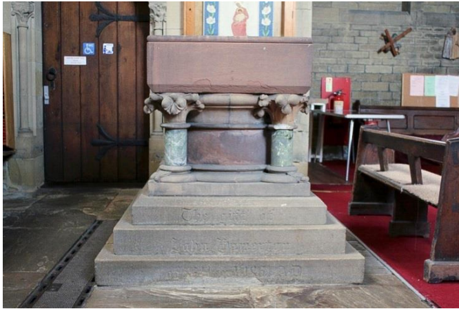
The font before cleaning, note how it was uniformly dirty, particularly the lower four courses.
