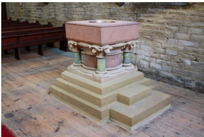
Another three-quarter view showing the historic, chronic soluble-salt activity in the masonry in the background. The new sandstone plinth blends in well with the bottom bed of the stepped base, but is likely to be obscured by future composite layers of under-floor heating.
