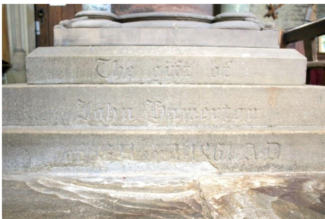
A detail of the historic efflorescence in the paving beneath the bottom step of the plinth, which has adversely affected the upstand of the bottom course. There was little point de-salinating this course, which is likely to have exacerbated the problem with long-standing soluble salt activity and created a very different cleaning differential with other courses.
