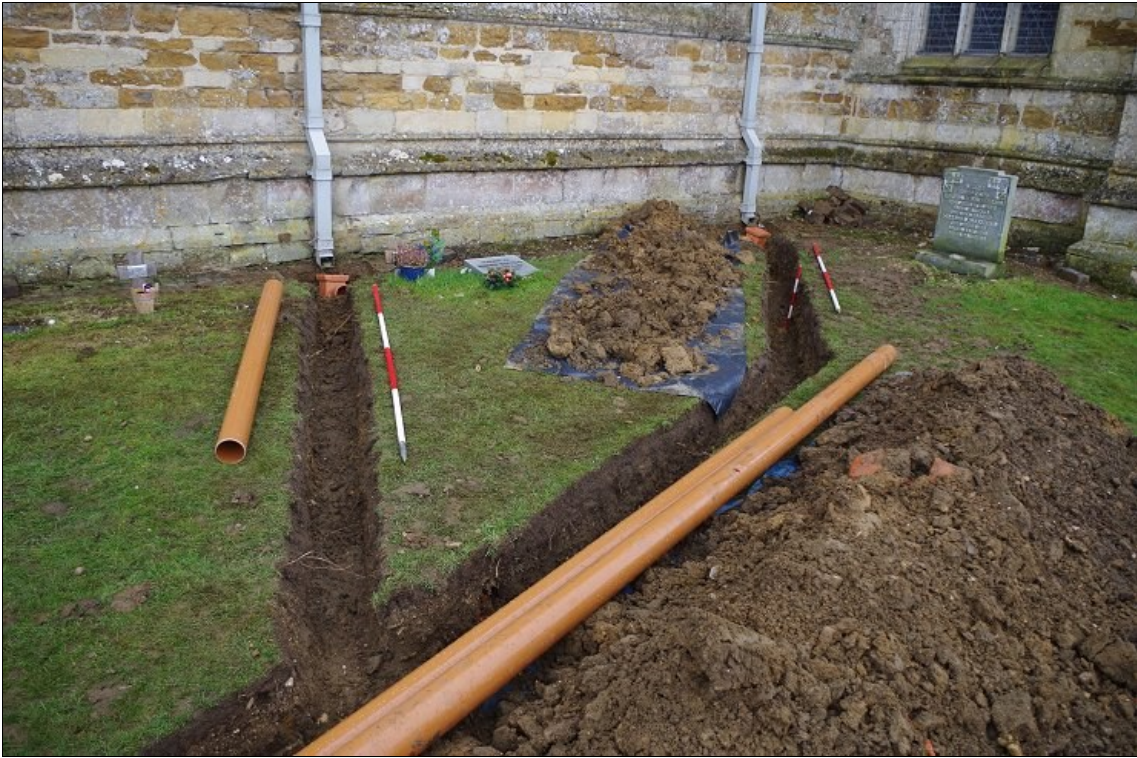
Photo 9. Part of Drain Trench 1 (on right) and Drain Trench 2 (on left), looking SW.
