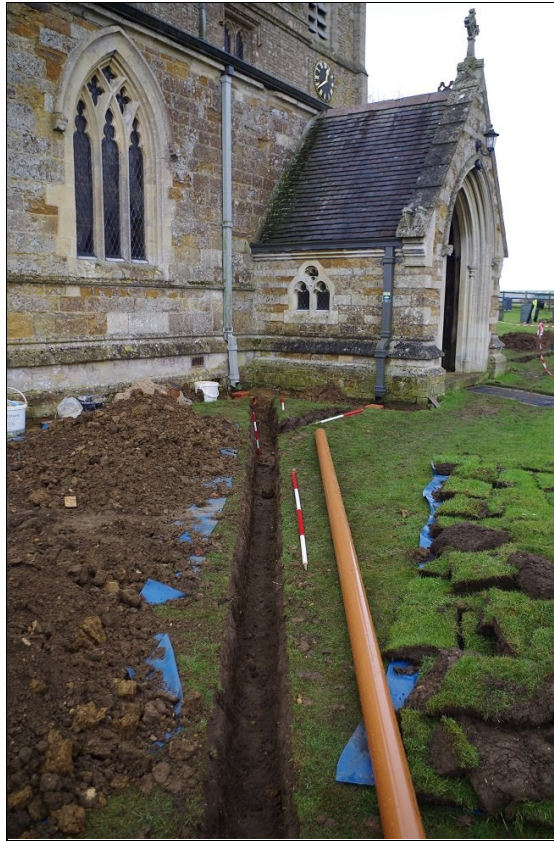
Photo 11. Drain Trench 3 (centre) and Drain Trench 4 (on right, by porch), looking SW.
