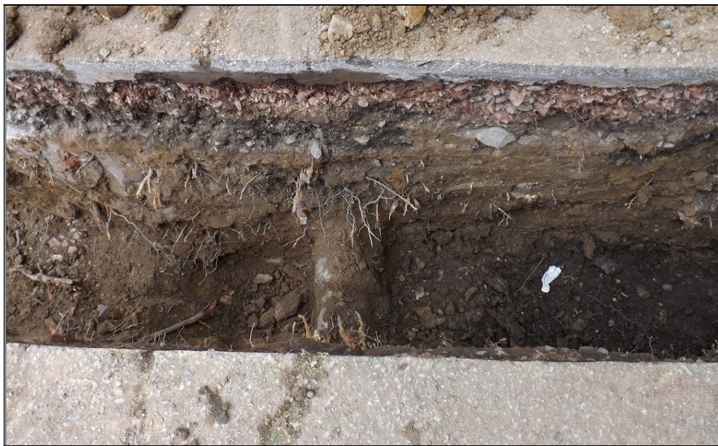
Plate 2. Typical deposits along the drainage run
