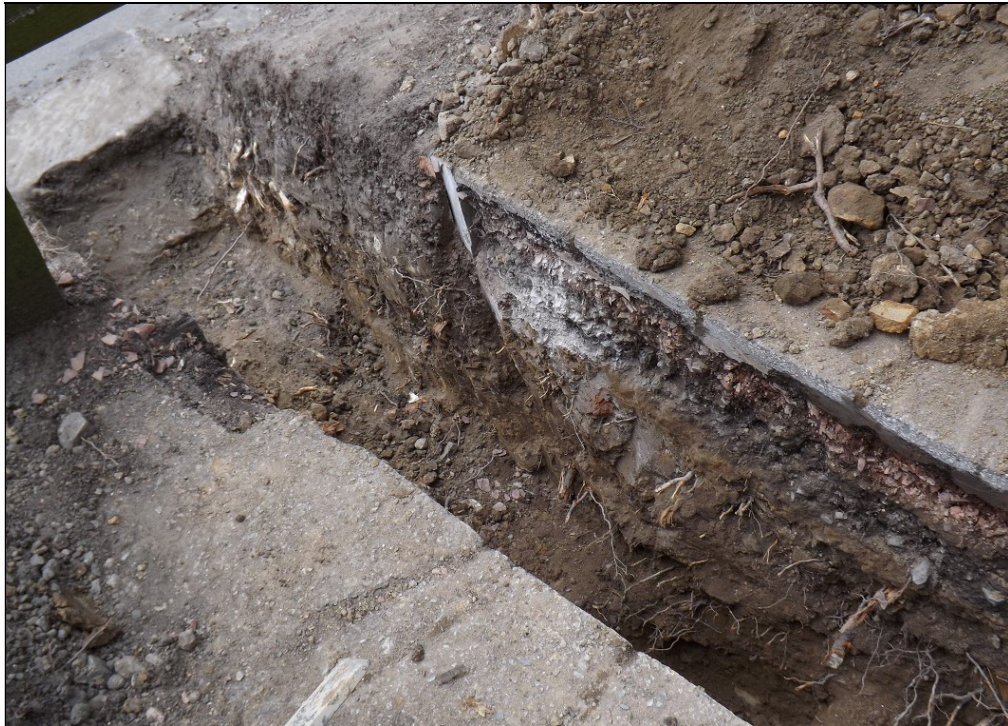
Plate 3. Typical deposits along the drainage run
