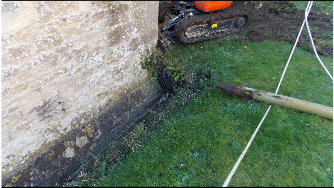
Figure 1. Existing stone drainage channel & vegetation covered void.
