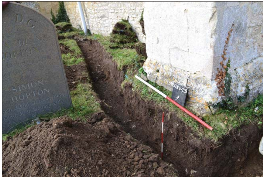
Plate 3. Hand dug trench against south nave wall and butress, looking north west, Scales: horizontal 1m and vertical 0.5m.
