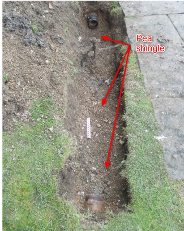
(Fig 5 – trench looking south-east showing compact layer of pea shingle following removal of collapsed drain)
