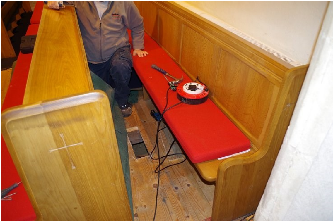
Photo 7. Intervention 3: Opening in floor of choir stalls on south side of chancel, looking SE.
