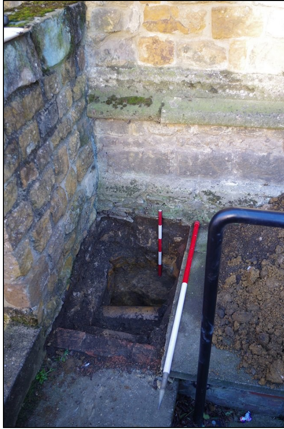
Photo 11. Intervention 7: Trial pit against exterior of north wall of north aisle, looking S.
