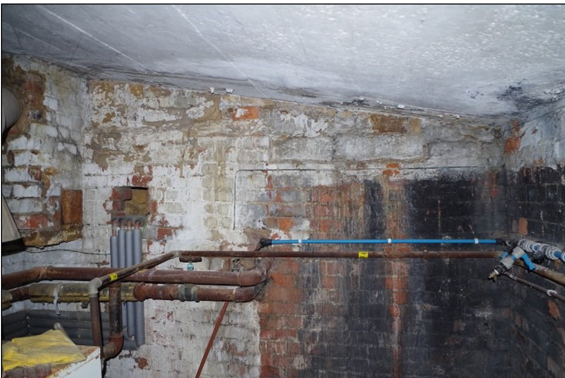
Photo 18. Brick-built west wall of boiler house underpinning stonework of east wall of north porch, looking W.
