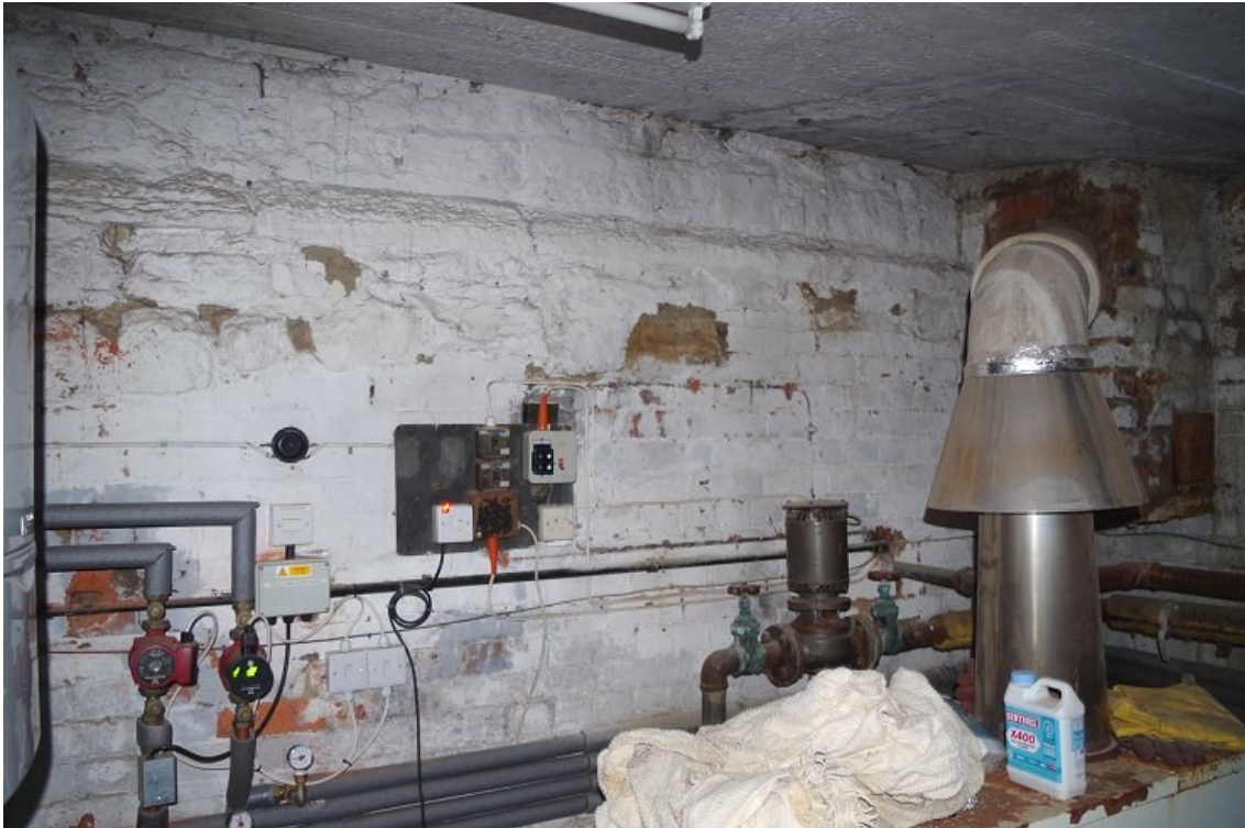
Photo 17. Brick-built south wall of boiler house underpinning stonework of north wall of north aisle, looking SW.
